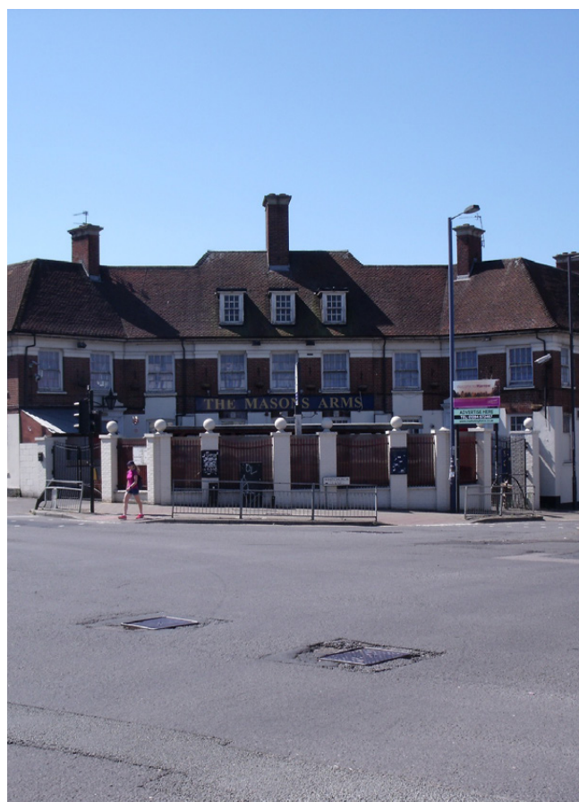
Figure 13 – The Masons Arms - a listed heritage building in poor condition
